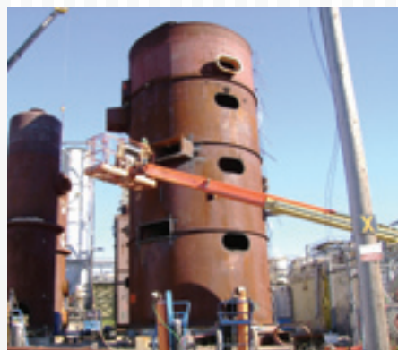
Fabricating the new converters, The Roberts Co. provided their valuable services to the project.
