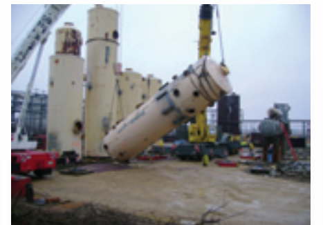
Oldies but goodies, towers from a Wisconsin-based U.S. army plant were incorporated into the Wilbara facility's modern design.
