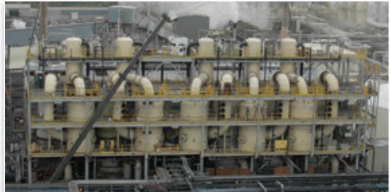
Plant expansion completed in six months, start to finish. The Roberts Company provided engineering, fabrication, and construction.
