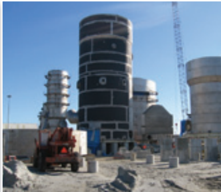
Sulfuric Acid Plant under construction—Towers fabricated and erected by The Roberts Company
